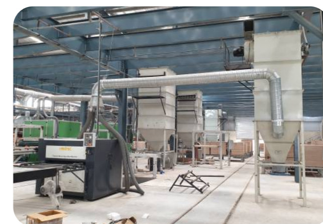
Dust Collector on Brushing & Sanding Machines
