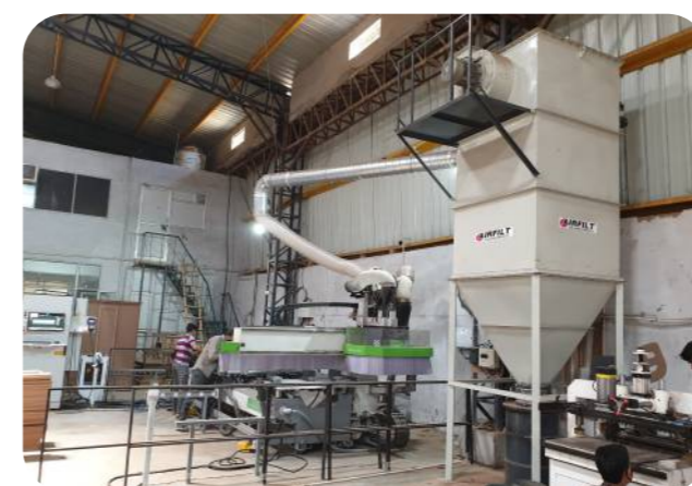
Dust Collector on CNC Router (Biesse)
